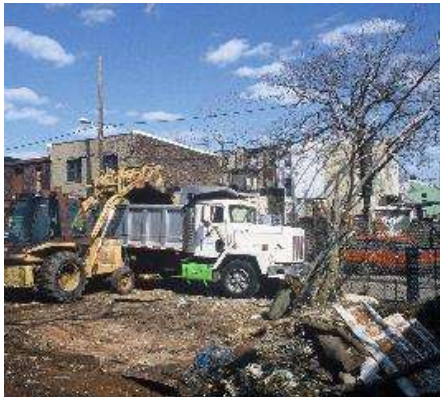
Major trash, debris, and weed removal
